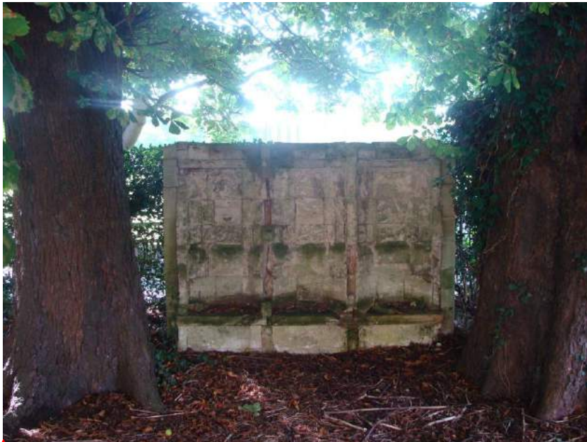
Picture 43 – 14 th century grade II Sedilia removed from church during 19 th century 'restoration', now in need of urgent repairs. Included on the Council's BuildingsHeritage at Risk Register.
