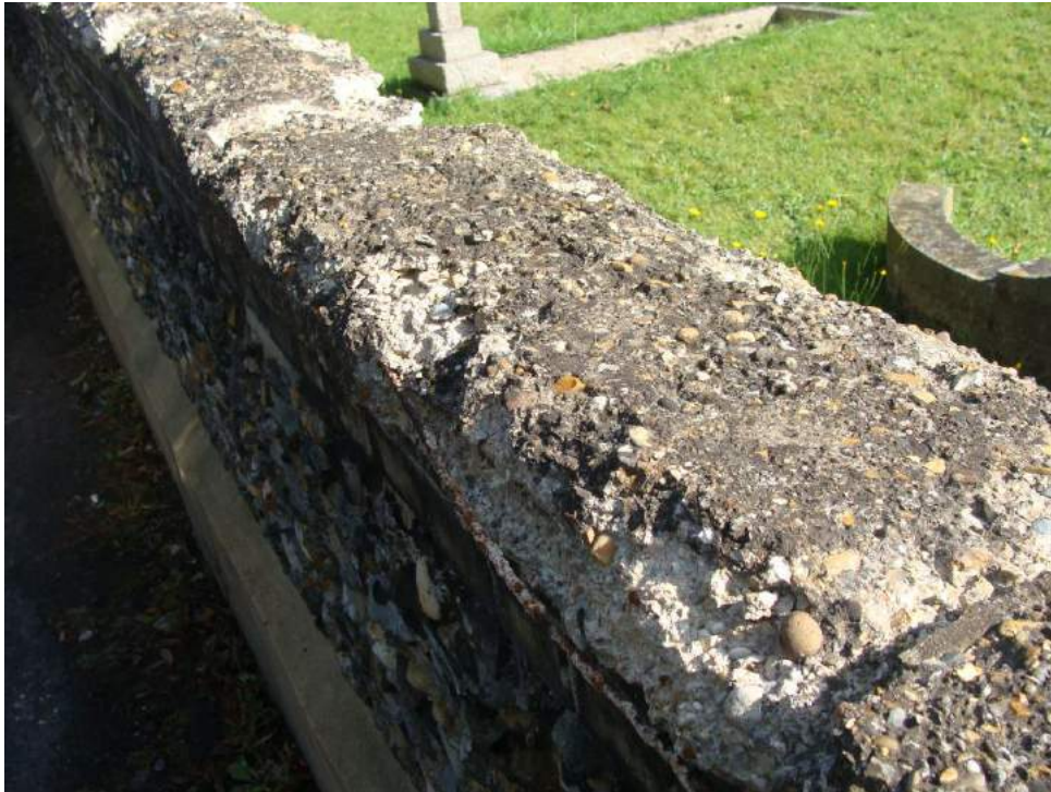
Picture 132 – Concrete capping slabs to church boundary wall. Picture retained as an historic record. These degraded capping slabs have now been replaced. in need of replacement.
