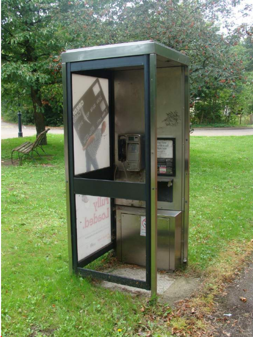
Picture 251 – Modern telephone box that should either be repaired or removed.
